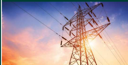
Electric Generation and Transmission
