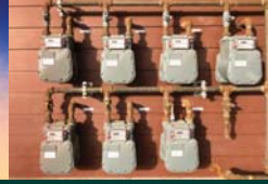
Natural Gas Transmission
